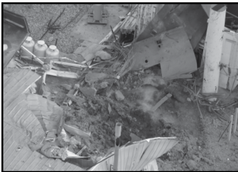
Figure #1: 20-foot diameter, 8-foot deep crater and structural damage caused by NO unit process explosion
