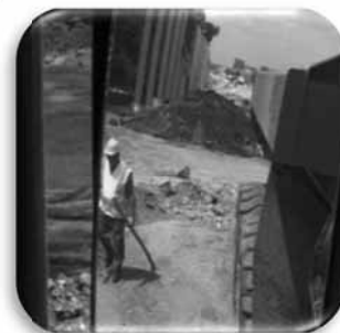
Adjust and clean mirrors; check back-up alarm.
