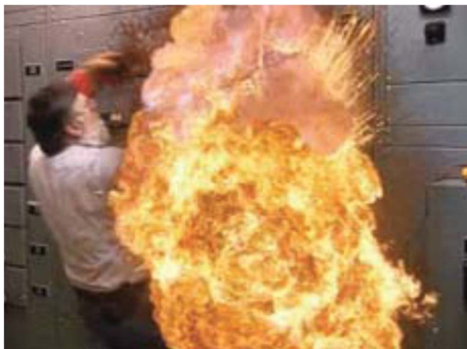
Photo of arc flash incident.
